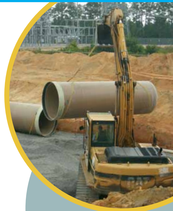
HOBAS pipe was used for fluid containment for an electrical substation
