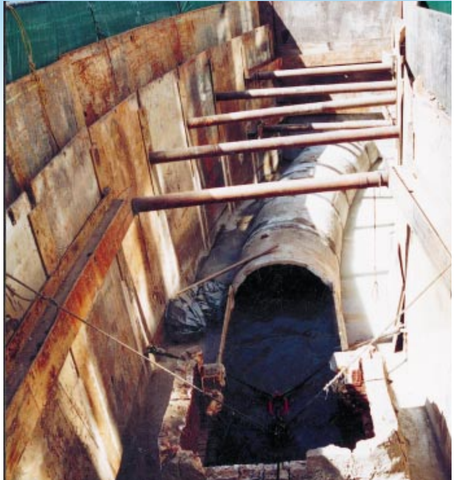
A section of the existing sewer was removed and this area was utilized as an insertion pit for curved sections.
