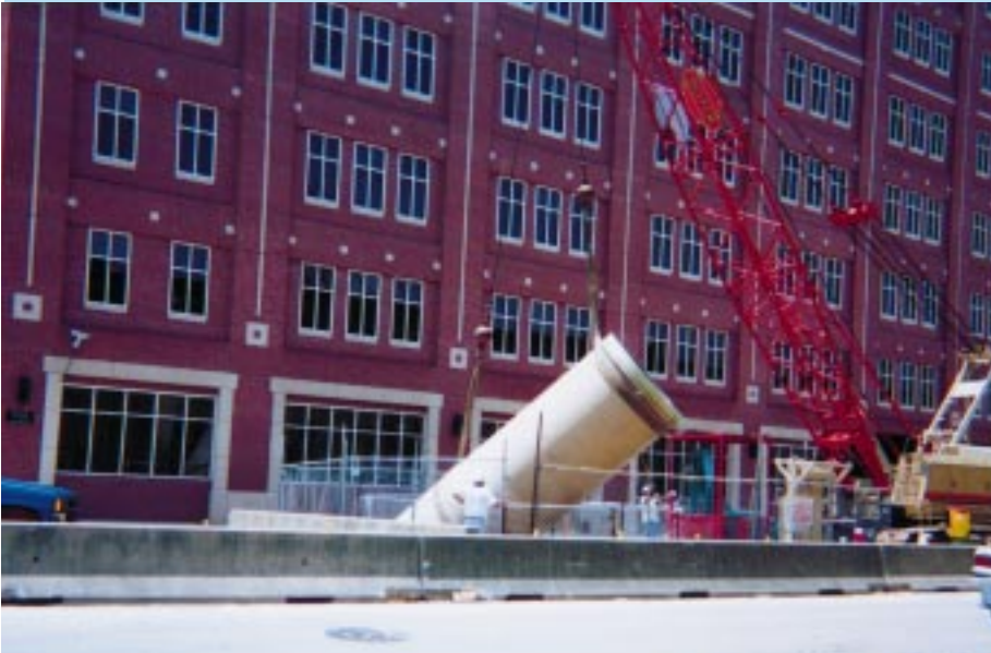
The pipe was installed adjacent to streets and buildings as well as directly below the bayou.
