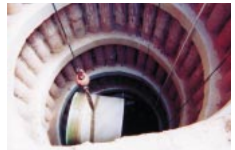
Short sections were fabricated to fit easily into small but deep shafts.
