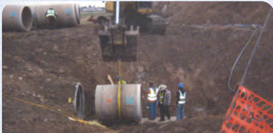
HOBAS PROVIDED MITERED FITTINGS TO EXACTLY FIT THE ALIGNMENT OF THE EXISTING WATERLINE UNDER RUNWAY 13/31.
