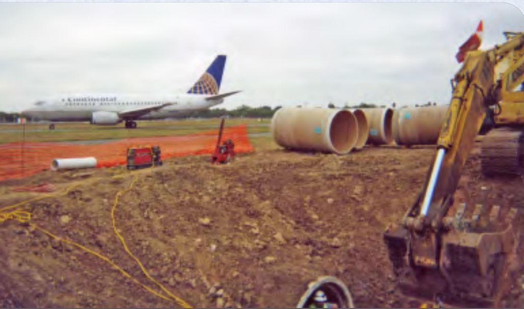
WORK WAS JUST OUTSIDE THE OFA SO THE RUNWAY AND TAXIWAY REMAINED IN SERVICE.
