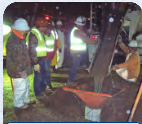
WORKING ON THE SURFACE AT NIGHT, THE CREWS COMPLETED THE GRAVITY GROUTING WITHOUT AFFECTING AIR TRAFFIC.
