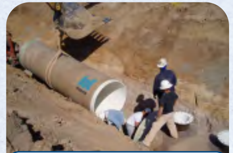
LIGHTWEIGHT HOBAS PIPES WERE QUICKLY AND SIMPLY INSTALLED. PUSH-TOGETHER COUPLINGS SPEED INSTALLATION.
