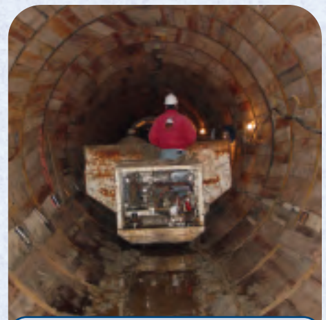
THE ENGINEERED PIPE WALL CROSS SECTION IS AN ADVANTAGE IN TUNNELS. IN MANY INSTANCES THE PRIMARY TUNNEL DIAMETER MAY BE DECREASED.
