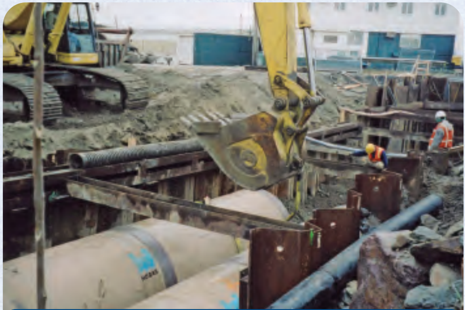
AT SUFFOLK DOWNS THE HOBAS CCFRPM PIPE IS INSTALLED BY DIRECT BURY IN A TRICKY TWIN BARREL CONFIGURATION.
