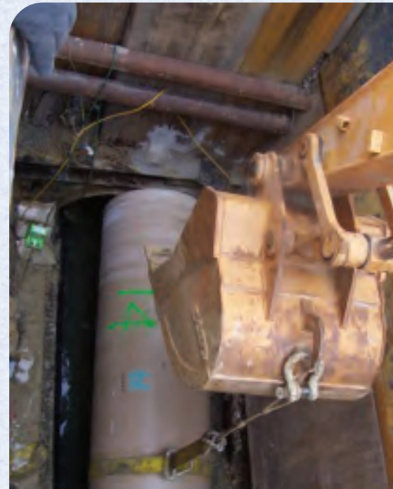
A SLING ATTACHED TO AN EXCAVATOR EASILY HANDLED A LIGHT-WEIGHT 20-FOOT JOINT OF HOBAS 48-INCH CCFRPM SLIPLINING PIPE.
