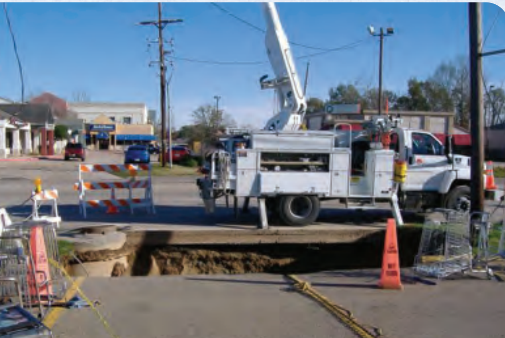
A SINKHOLE FORMED IN BATON ROUGE ALONG THE SHOULDER OF ESSEN LANE.
