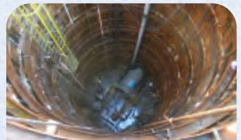
ANOTHER SECTION OF HOBAS PIPE IS INSTALLED AT THE BOTTOM OF A 70-FOOT PIT, ONE OF THE DEEPEST USED DURING THE CLEVELAND PROJECT.
