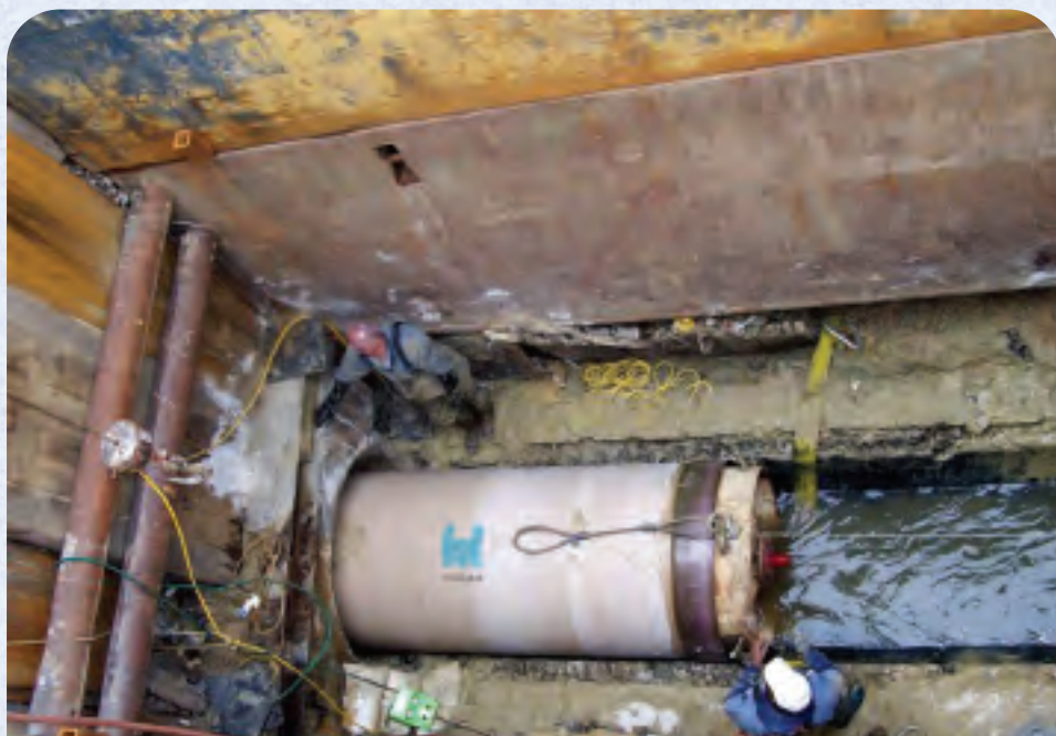
ALLEN & LEBLANC CREW MEMBERS SLIP THE 48-INCH HOBAS CCFRPM PIPE INTO POSITION WHILE MAINTAINING FLOW.
