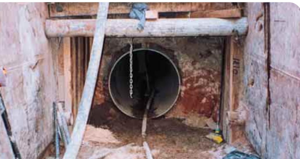
THE HOBAS PIPE WAS INSTALLED DIRECTLY WITHIN THE ROCK TUNNEL AT DEPTHS OF UP TO 50 FEET.
